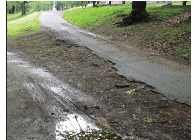
Erosion of asphalt paths at low point in lower terrace area
