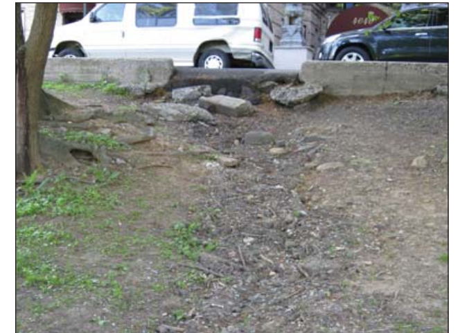
Deterioration of raised curb and slope erosion at Bronx Blvd.
